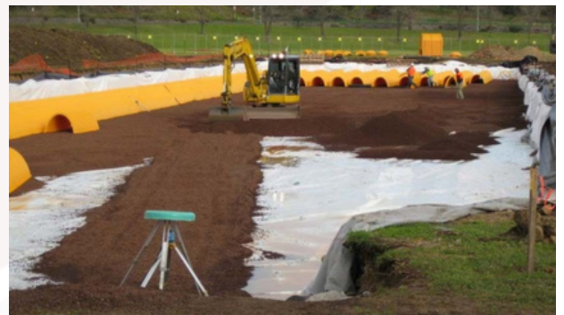
The additional storage tank built in 2008 is located under a sports field (Photo courtesy of City of Melbourne)
