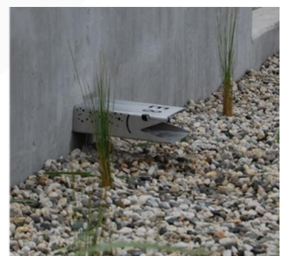
Stainless steel eel-head spout directs stormwater into the raingardens
