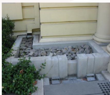
Prior to entering the raingardens, roofwater is directed into a small detention system to reduce flow velocities
