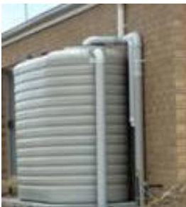
Rainwater tank on site
