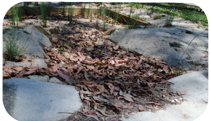
Blocked inlet, roadside infiltration basin, Mount Evelyn.
