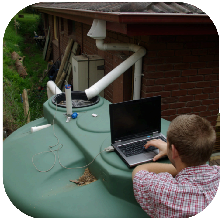
Monitoring levels of rainwater tanks
