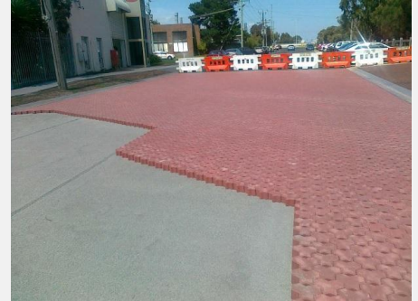
This site trials porous material on a road subject to heavy traffic volumes (shown here: interlocking pavers)
