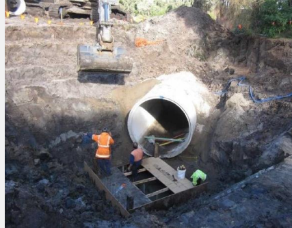
Underground pipes allow storage of 187kL
