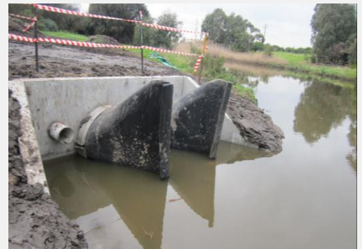
Tideflex valves prevent backflow from Mordialloc Creek into the storage area
