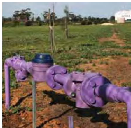
Figure 16 Recycled water meter assembly with purple to identify it contains recycled water.
