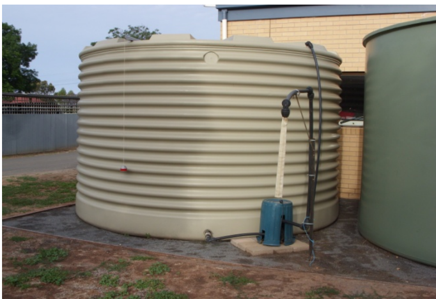
Figure 13 Storage tank for recycled water at Donald
