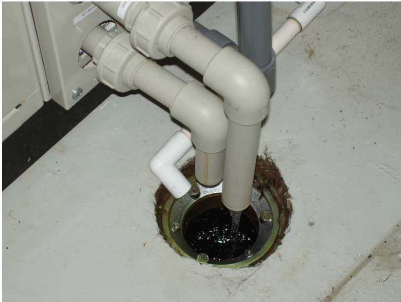
Figure 8 Discharge from central unit of RO reject water
