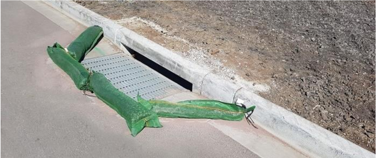
Figure 5.3. Silt sock in use to prevent sediment entering drain inlets. (photo courtesy of McConnell Dowell)
