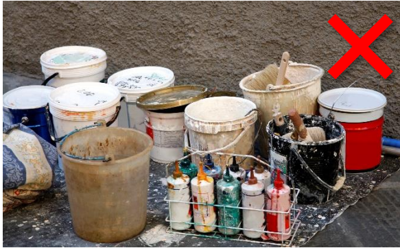
Figure 7.1. Incorrect chemical storage onsite.
