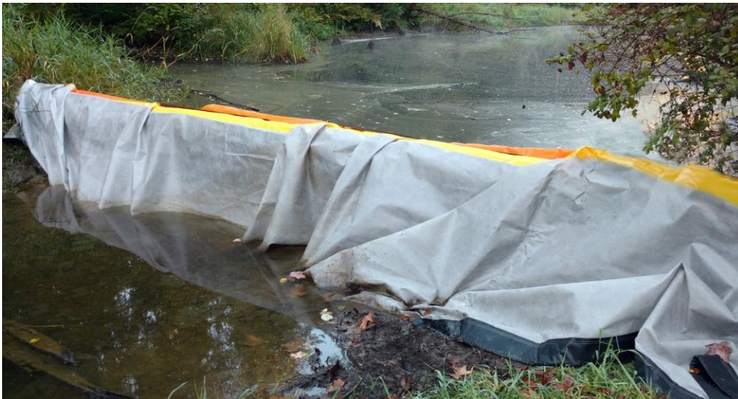
Figure 1. Engineered silt curtain installed to prevent migration of sediment for construction works within a waterway.
