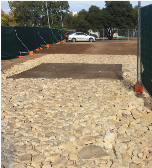
Figure 2. Rumble grid. (photo courtesy of McConnell Dowell)
