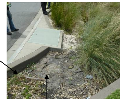
Erosion and scour from high flows
